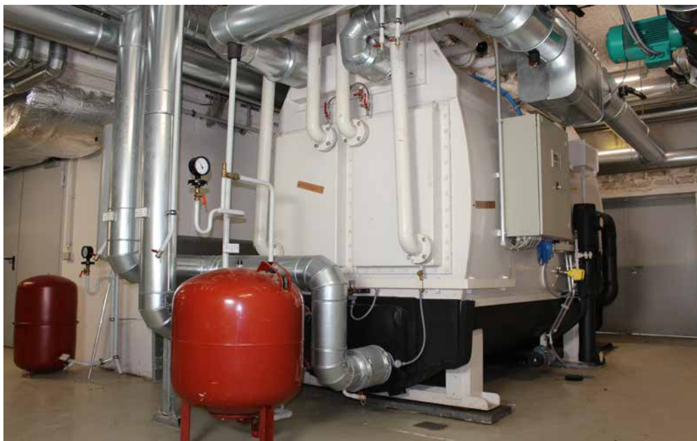
Adsorption cooling machine at the Environmental Campus
