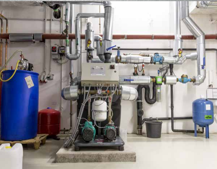
Control centre for the rainwater system
